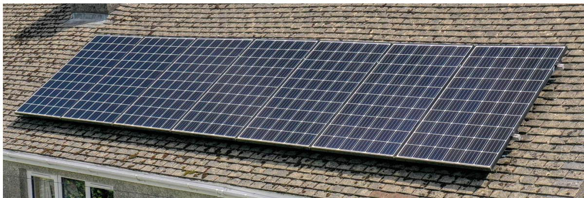
Figure 59 Roof-mounted system (EnergyCC, 2020)
