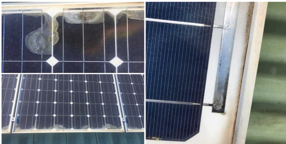
Figure 17 PV panel water vapour ingress effect ( Review, 2018 )
