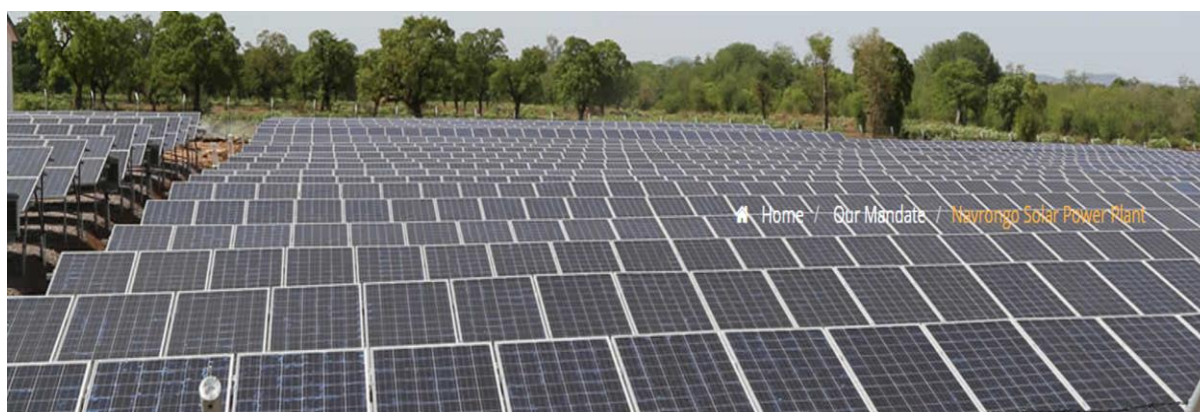
Figure 24 2.5MW Navrongo Solar Power Plant (VRA, 2018)
