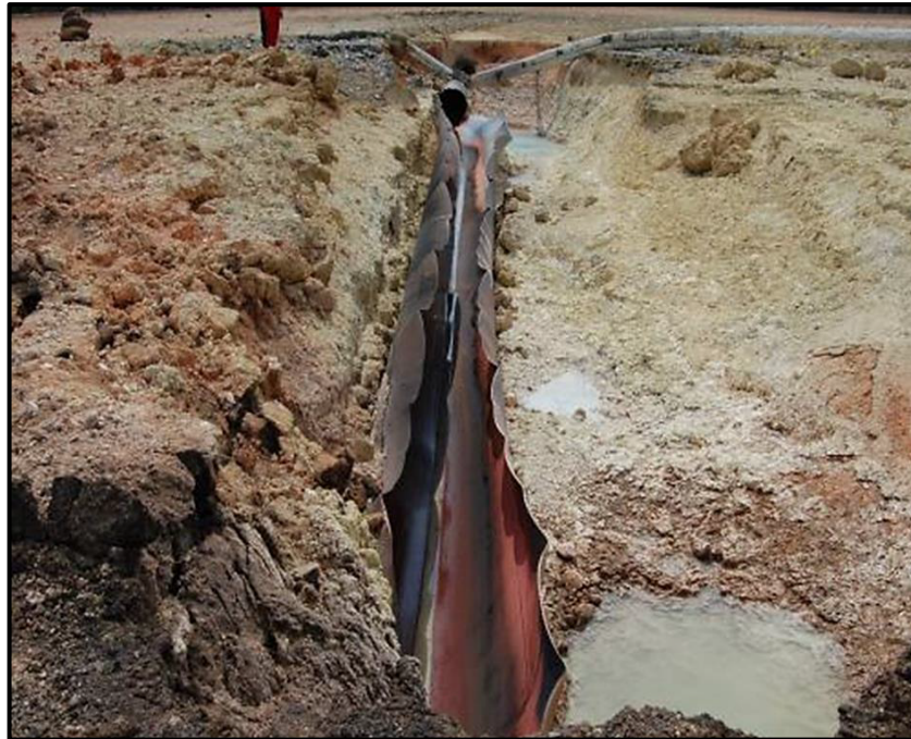
Figure 4.7 – Ruptured Section of Pipeline (Texas 2010) (NTSB, 2013: 8)
